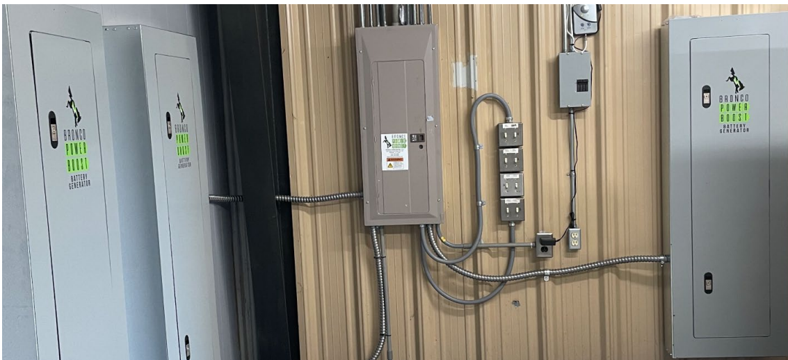
Nanney Civic Center Back-up Power for 15,000 square foot facility
