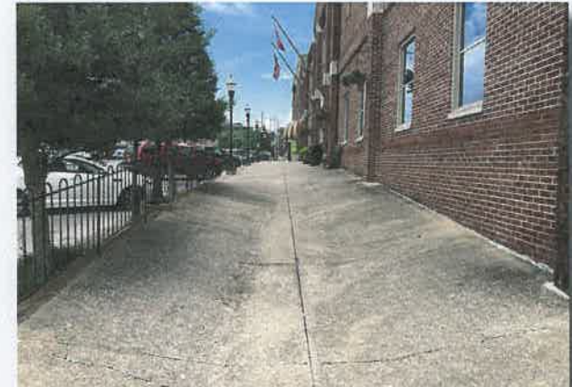
The segment of sidewalk in front of City Hall on the east side of the Square features a concave surface. That situation should be rectified with a new streetscape design.
