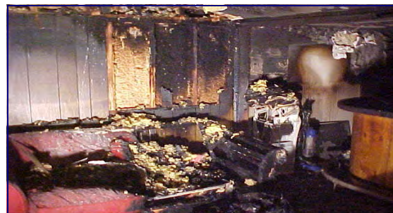
Damages after the fire on Fischer Drive
