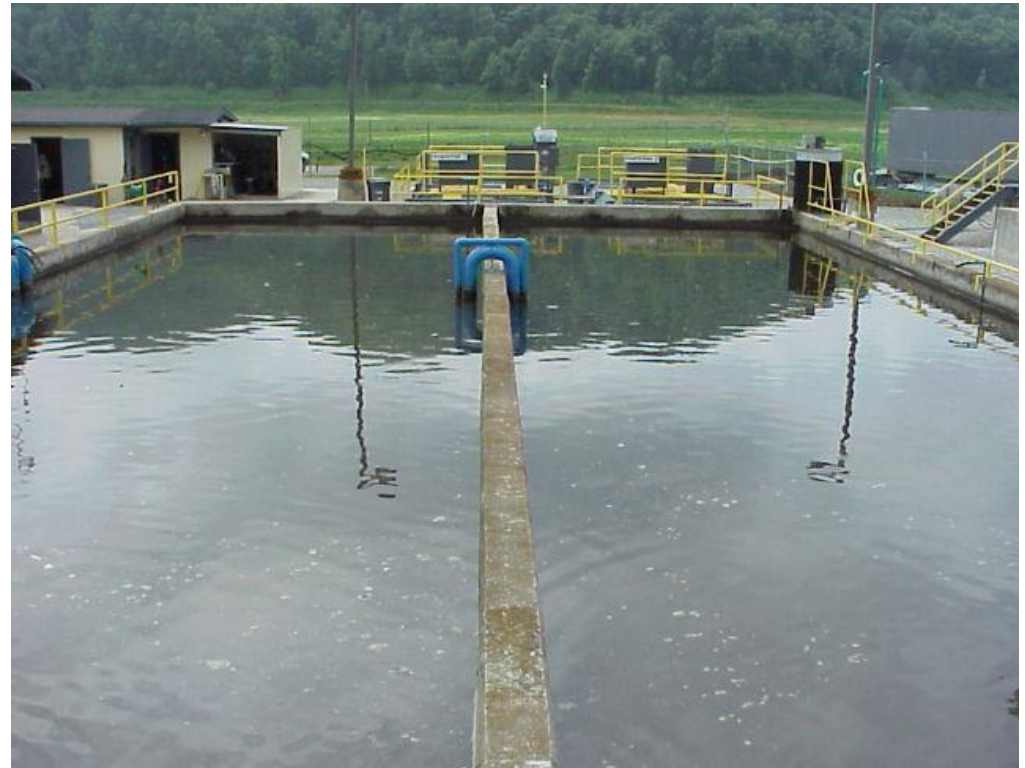
Aerators with air “off”
